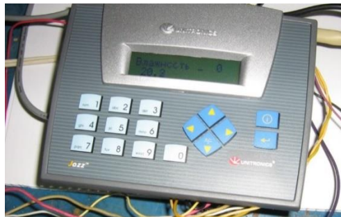
Figure 7 – The PLC screen showing the humidity level value
